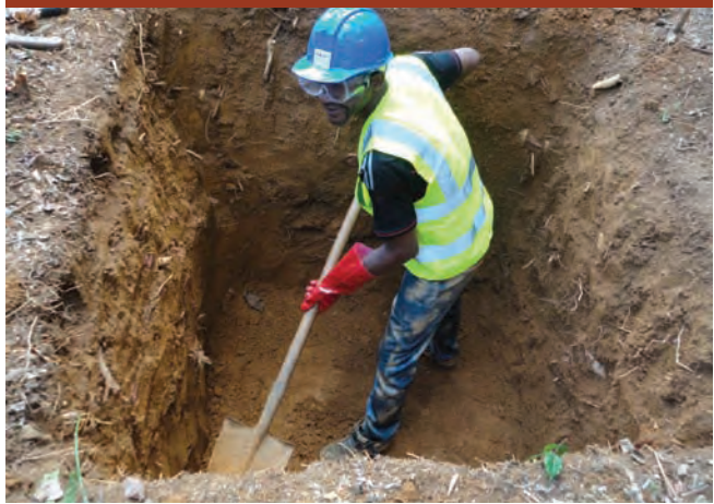
Pitting at Nayega, Togo
